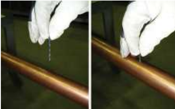
Clean spraying holes
